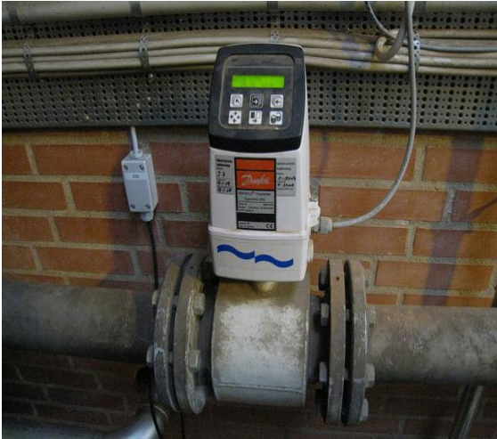
The flow meter
